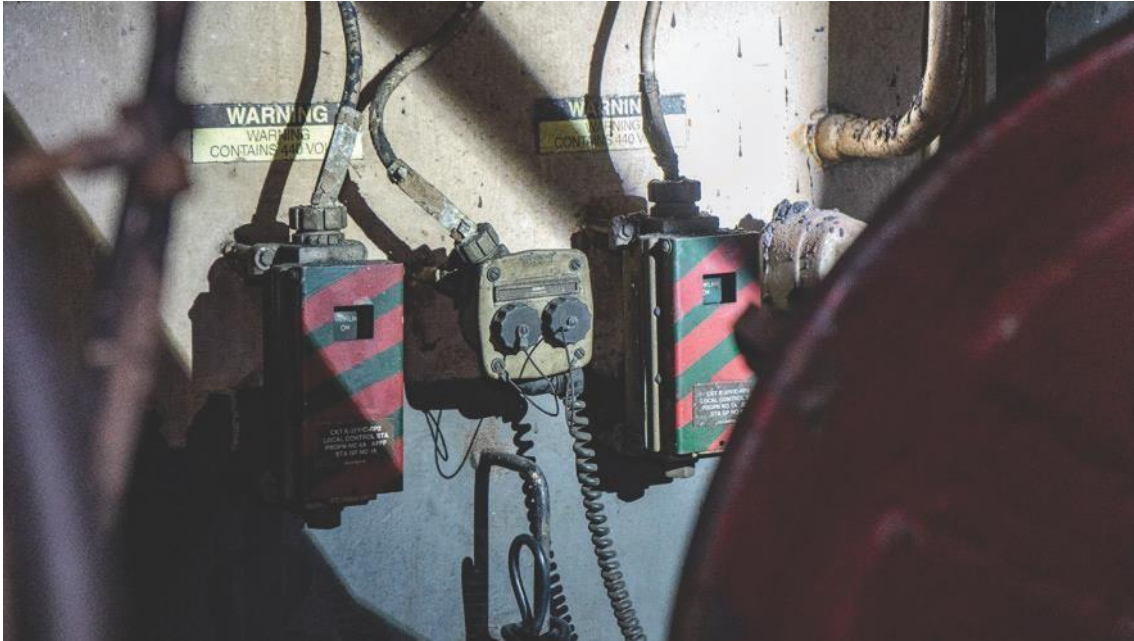
79 Figure 30, Still photo of AFFF push-buttons for sprinkler groups 15 and 16 serving Lower V with covers closed (16 on left; 15 on right). These push-buttons are in Upper V amidships. The photo shows proximity to open hatch, which obstructs visibility of the push
