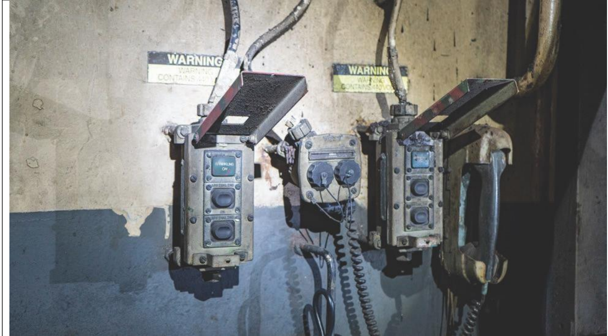
80 Figure 32, Still photo of AFFF push-buttons for sprinkler groups 15 and 16 serving Lower V with covers open (16 on left; 15 on right). These push-buttons are in Upper V amidships
