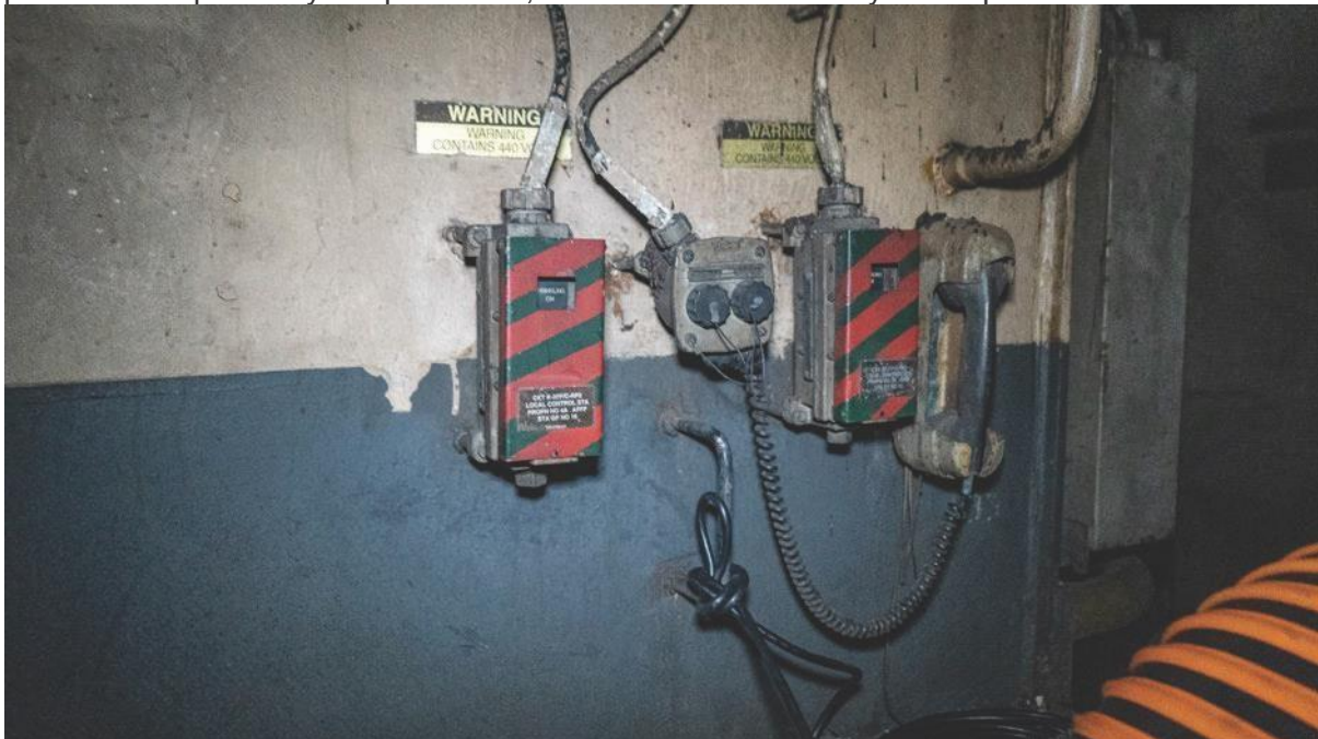
, Still photo of AFFF push-buttons for sprinkler groups 15 and 16 serving Lower V with covers closed (16 on left; 15 on right). These push-buttons are in Upper V amidships.
